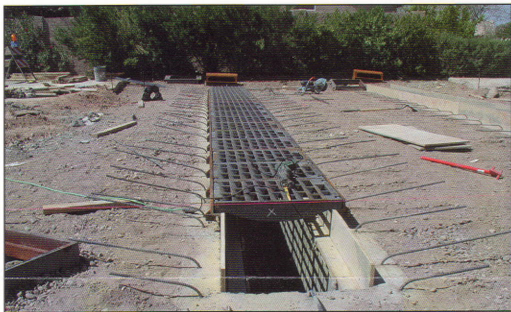
View of the concrete channel that sits below the grate and runs perpendicular to the roadway.
